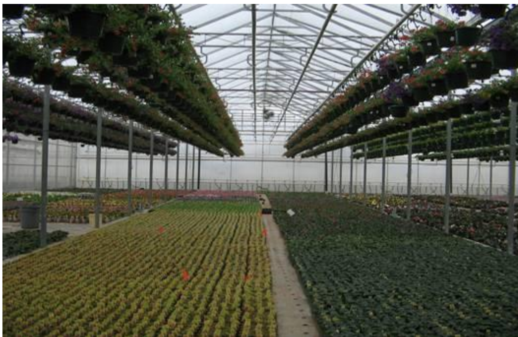
The above picture shows the overhead basket mechanization (computer controlled) at Rainbow Greenhouses. It allows for accurate measurement of water good enough for each basket plant thus, saves water. Watering takes place in one location, usually the walkway, so no baskets will drip on other
