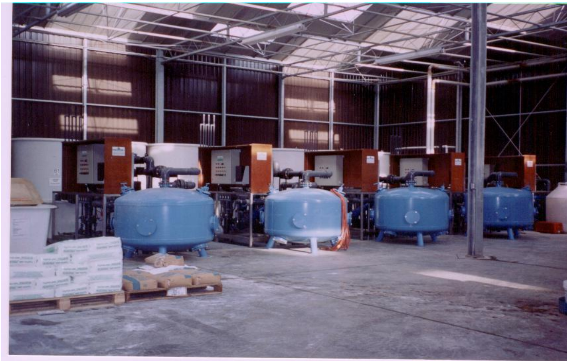
High speed sand filters (blue tanks) to reduce pathogens, thereby reducing use of chemicals.
